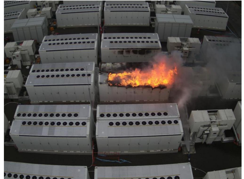
Fire events in battery plants
