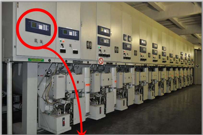
Control room of a substation
