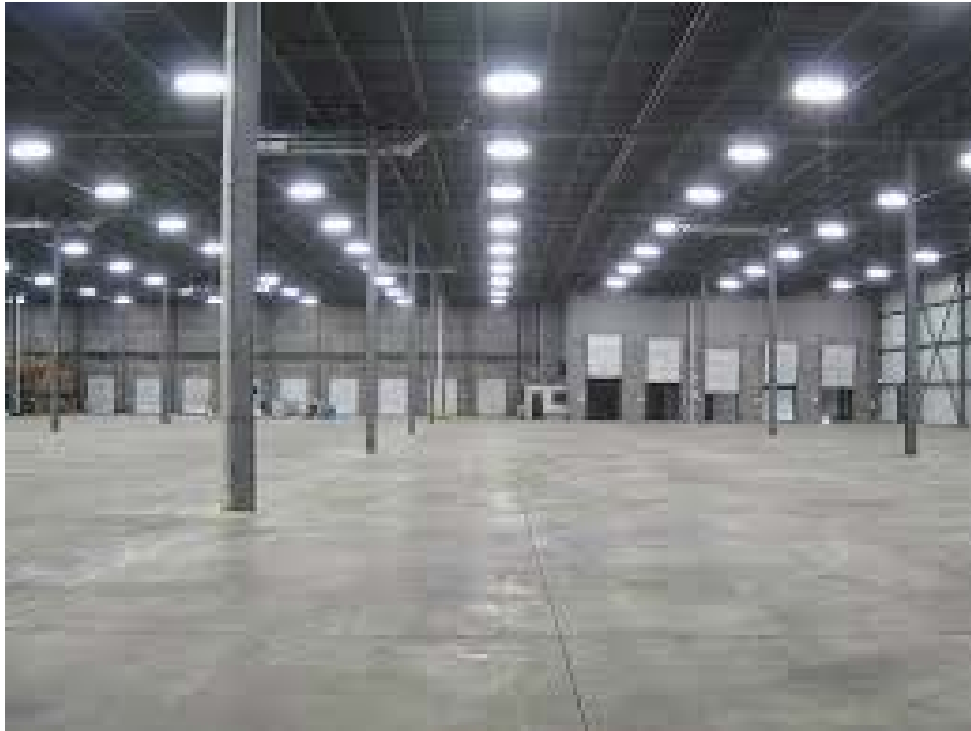
Example Photo: Commercial LED Lighting Retrofit
