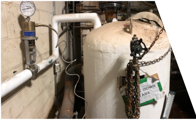
Blowdown tank, municipal water line, and temperature regulating valve that previously cooled boiler blowdown water before it went to the drain.
