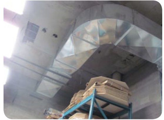
Duct work from the compressor brings warm air to different areas of the plant
