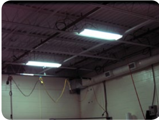
New T-8 lighting saves Jacobs & Thompson $3,220 per month in energy costs
