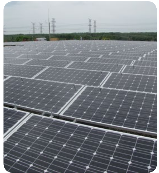
Veridian's rooftop-mounted solar array features over 400 photovoltaic panels
